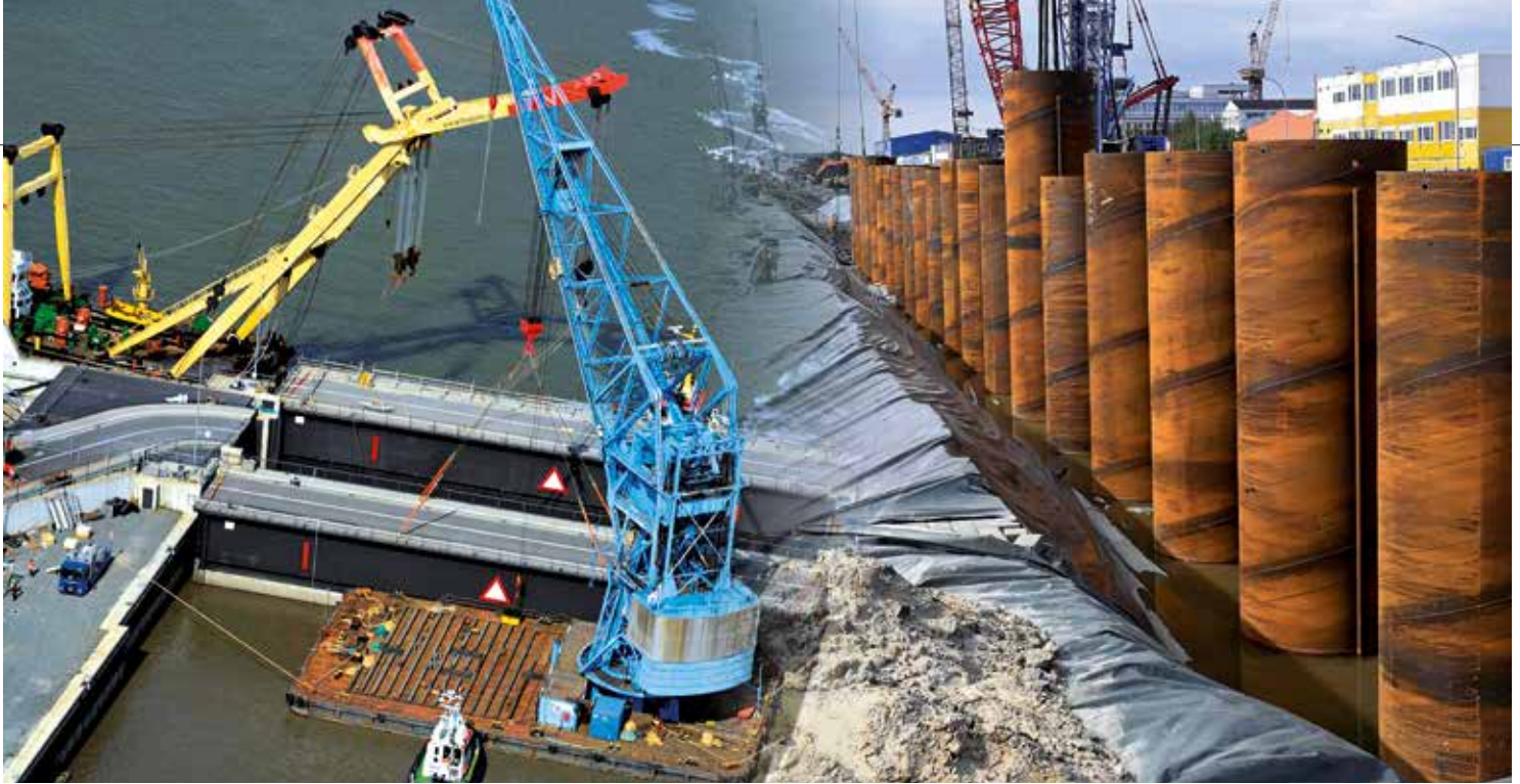
The Kaiserschleuse (l.) and Westkaje at the Kaiserhafen (r.) are just two examples of the many infrastructural measures in Bremerhaven.
