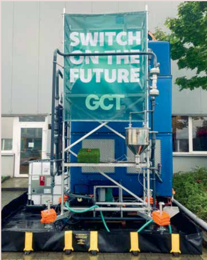
The DAC demonstration system in Essen boasts an annual capacity of 100 tonnes of carbon dioxide.
